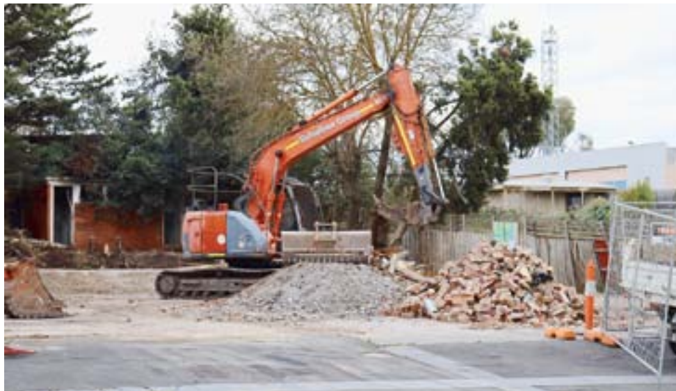
Machinery has been brought in to sort through the rubble of the old fire station building.
